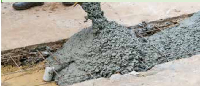
Wet concrete being poured onto steel reinforcement bars at a construction site © Shutterstock
